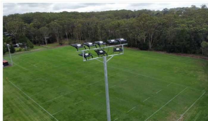
Figure 3: Sports field lighting LED upgrade at Yulong Oval, Medowie completed in 2023.
