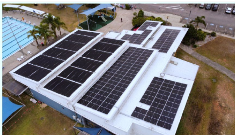
Figure 6: Solar PV and solar pool heating installed at Lakeside Aquatic Centre in 2024.
