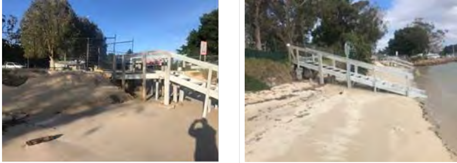
Before and after photos showing placement of sand to address undermining of stairs at Nelson Bay Beach. The sand was sourced via dredging of Little Bay boat ramp, where accreted sand was impacting the use of the boat ramp.
