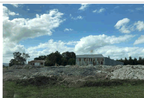
Photo 2: Looking North-East, approved mound being constructed, proposed site of development and existing metal shed
