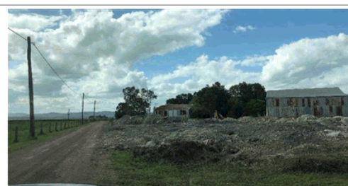
Photo 1: Looking North down Swanreach Road towards Hinton Road, approved mound being constructed and existing metal shed
