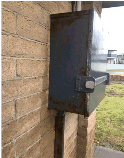
Figure 3 – Significant corrosion to switchboard. Asbestos backing board within switchboard.
