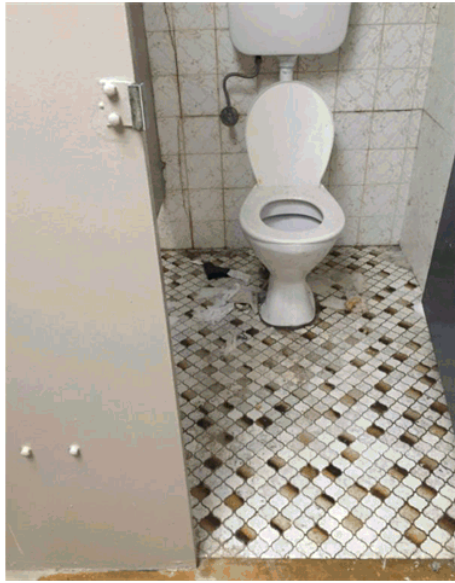
Figure 5 – Vandalised ceramic toilet currently out of commission.
