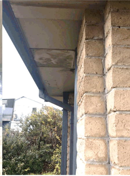
Figure 2 – Asbestos eave lining through out current building
