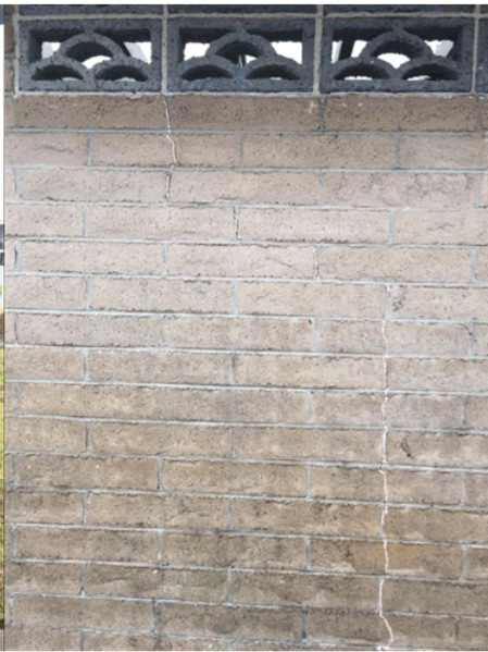
Figure 4 – Significant vertical and horizontal cracking in wall structure.
