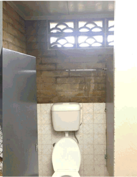
Figure 6 – Horizontal cracking in wall structure with clear daylight between brickwork.
