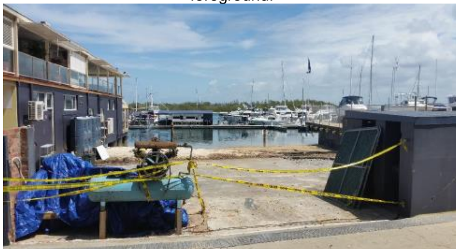
Image 5: Photograph of the existing slipway. Facing west from ground level showing the current site conditions.
