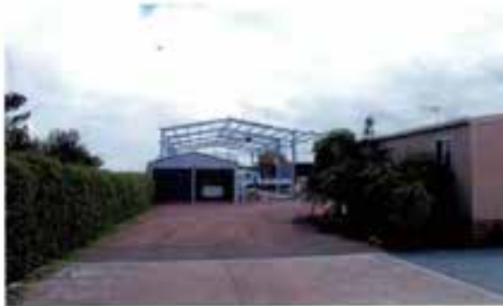
Photo 1 – The steel framework of the partially constructed rural shed viewed from the rear of the existing residence.
