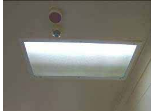
Picture 4: Light fitting recessed & flush to ceiling
